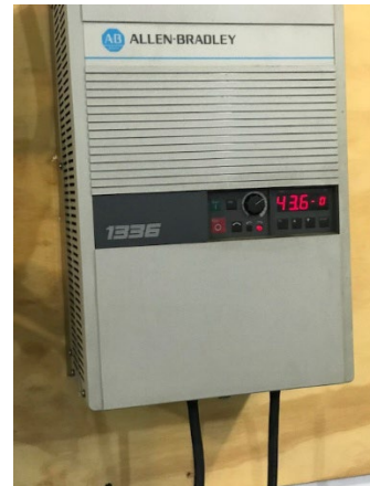
Allen-Bradley drive used for testing purposes.
